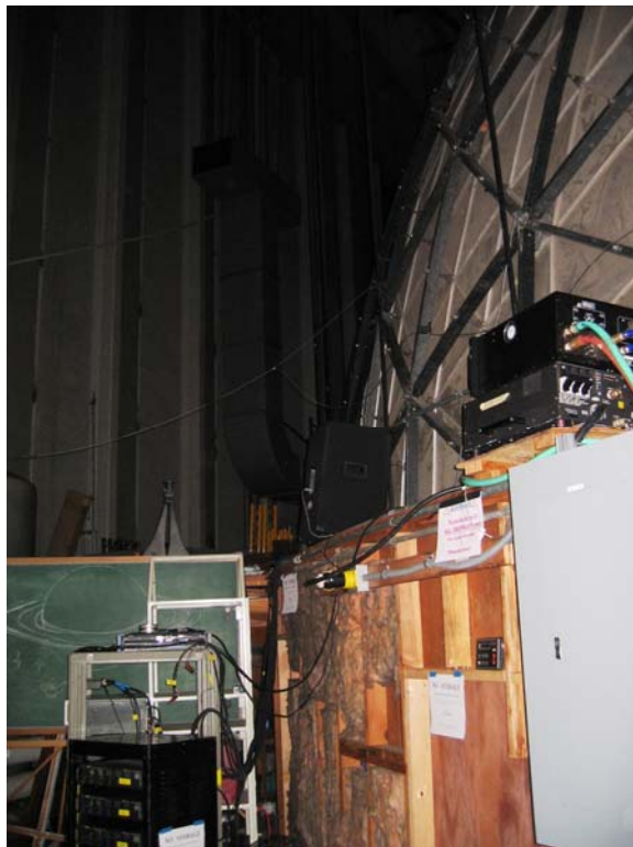
Figure 53 – Laser Dome (1962: Building 3) theater; view of dome structure from interstitial space storage
