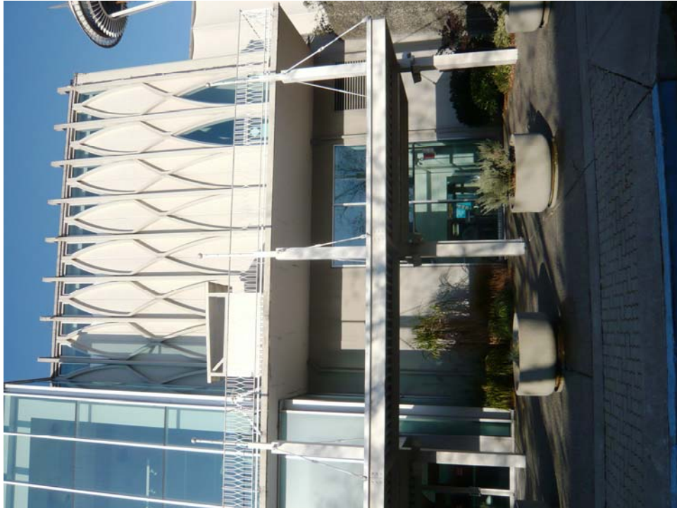
Figure 88 – South elevation of Building 3 (1962: Building R), east part. The steel walkway canopy structure and large glazed bay dates to 1992-93 renovations. Railing and balcony at middle of picture, as well as glazed openings at and between arches are original to 1962 building.
