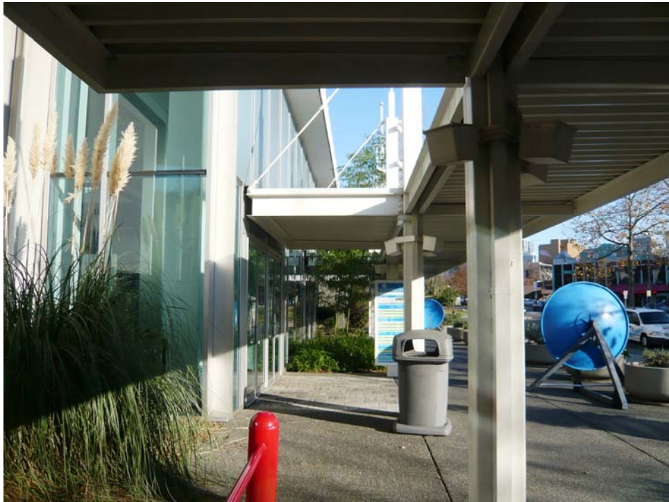
Figure 86 – Detail, south elevation Building 3 (1962: Building R). The steel walkway canopy structure dates to 1992-93 renovations to create a south entry at Denny Way.
