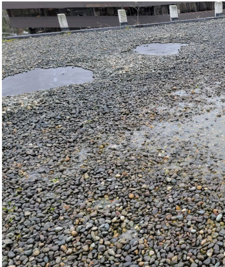
Ponding Water on Roof
