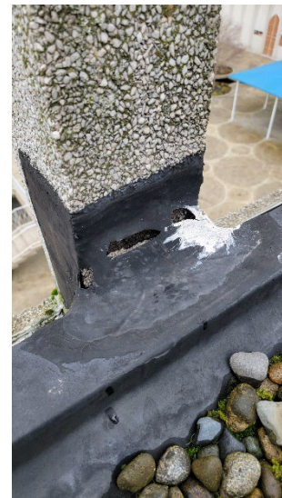
Roof Seal Damage
