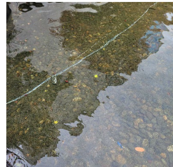
Joint @ Pool Bottom
